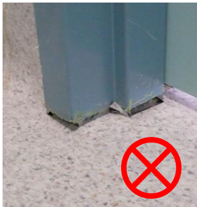
Figure 28: Gaps between door frame and floor
