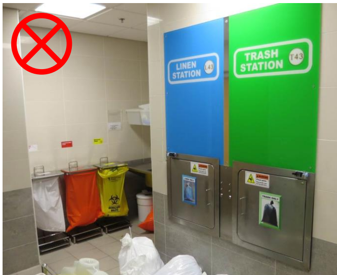
Figure 16: Linen and Waste chutes are not permitted
