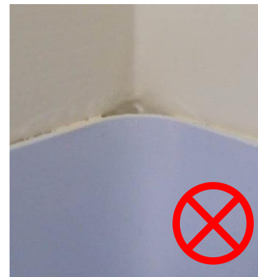
Figure 30: Gap between skirting and walls
