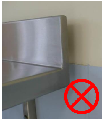
Figure 29: Gap between bench fitting and wall
