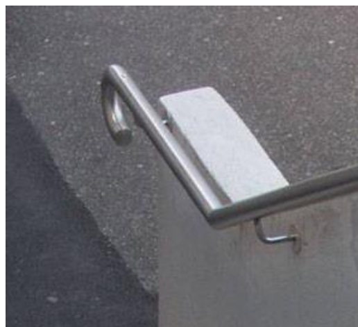
Figure 7.6: Compliant, rail extends beyond the stair
